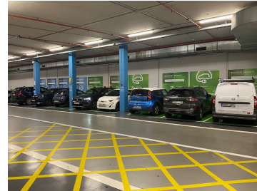
electrical terminals in Spain
